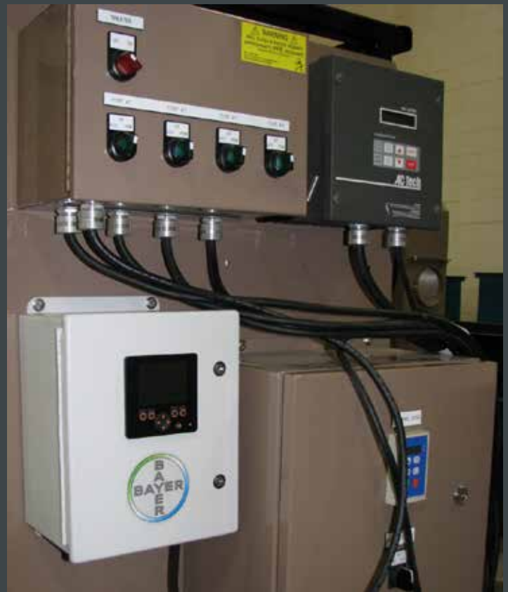
Flow Meter installed on old style 3-piece RH 4-pump control panel
